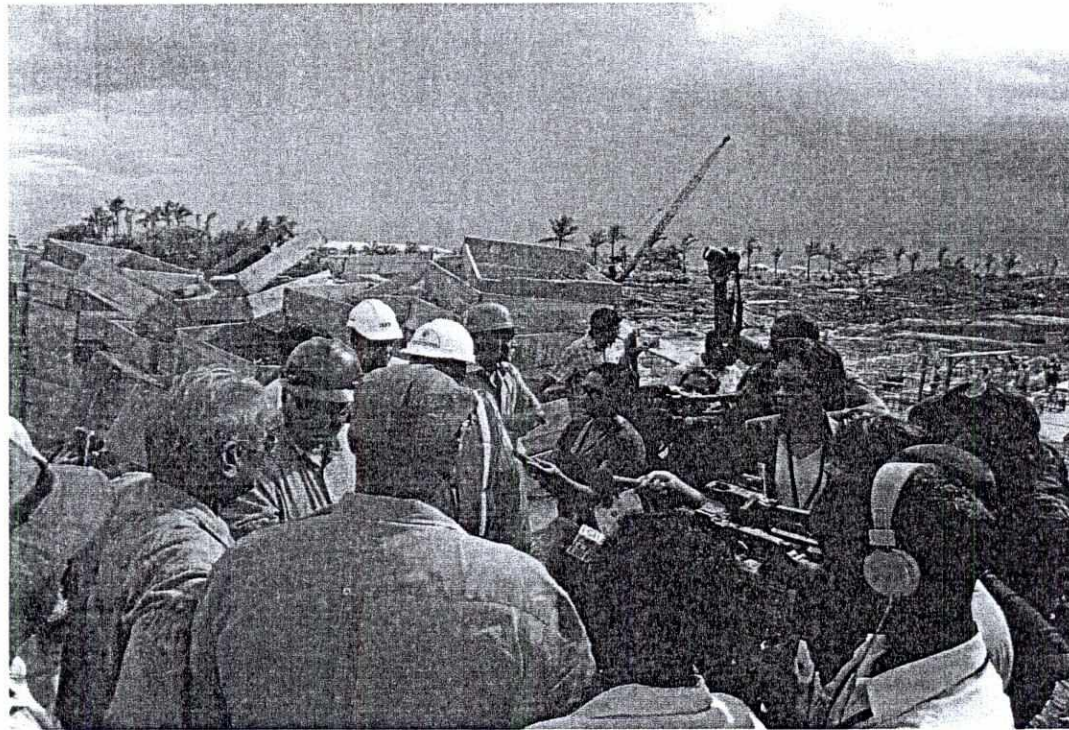
Members of the Delegation being brief on the progress of the High Level Outfall Sluice
