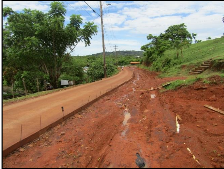
No reinforced concrete drains constructed and only half of the reinforced concrete payment completed - 15 August 2019
