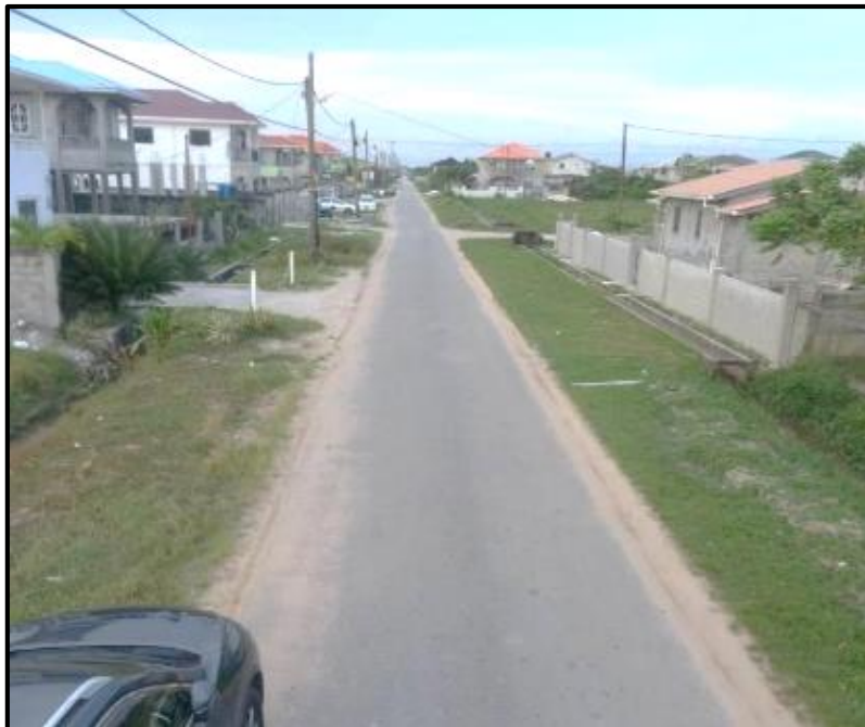
Condition of the road at 1 st Avenue, La Parfaite Harmony for which the contract was signed to rehabilitate - 8 October 2020
