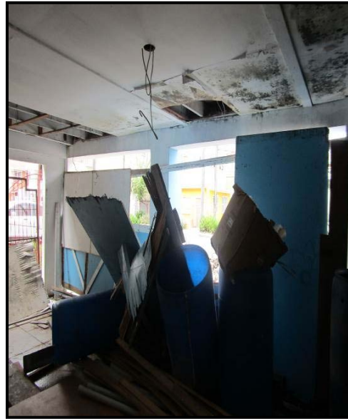
Fixed glass shop front windows not installed
