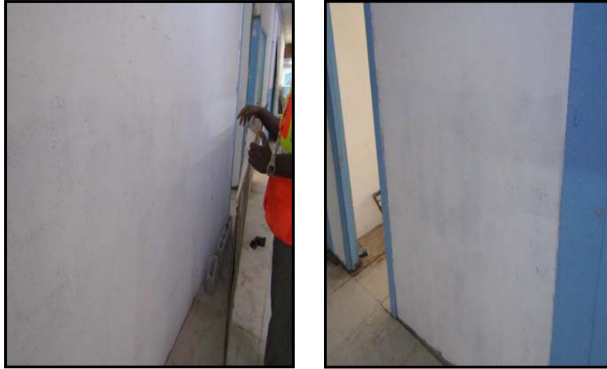
Poor quality of painting work observed
