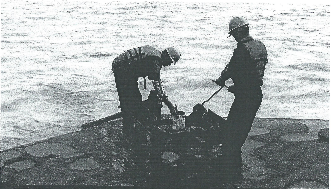
OPERATIONS MAINTENANCE STAFF TREATING CORRODED AREAS ON ANCHOR CHAIN
