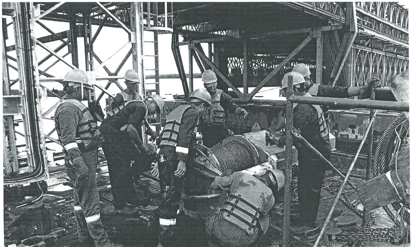
(ABOVE & BELOW) OPERATIONS MAINTENANCE STAFF REPLACING THE SOUTH EAST MAIN ALIGNMENT WINCH WIRE ROPE ON THE EAST RETRACTOR SPAN
